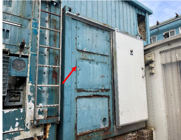
Photo 122: Get Fish, exterior, eastern area, shipping container – lead based blue paint
