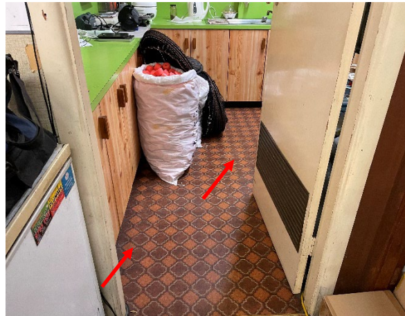
Photo 29: Internal, Net & Tackle level 1, kitchen floor – asbestos-containing fibrous backing to non-asbestos vinyl floor sheeting
