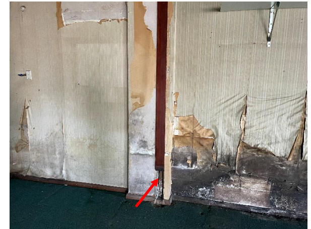
Photo 114: Net and Tackle, internal, level 1, south wall, formwork – asbestos containing fibre cement debris
