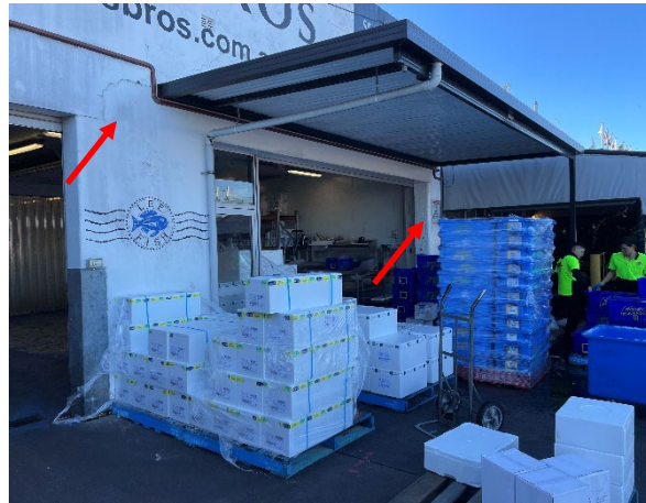
Photo 59: External, Poulos Bros, wall – lead based white paint
