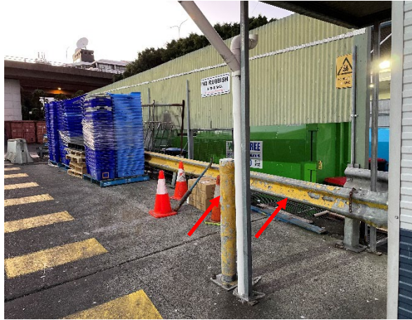
Photo 86: External, traffic bollards and fence – lead based yellow paint
