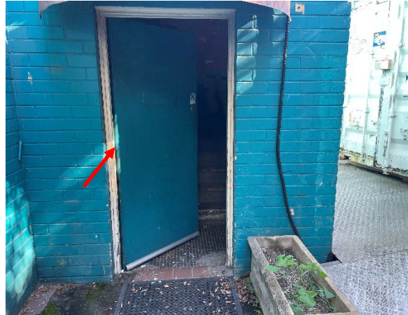
Photo 116: Net and Tackle, external, door frames – lead based cream paint
