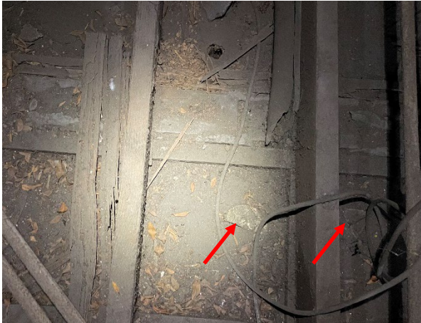
Photo 31: Internal, All Seas, ceiling cavity – asbestos containing corrugated fibre cement sheet debris
