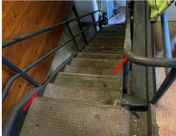
Photo 20: Internal, Doyle's Warehouse, stairwell and handrail – lead based blue paint
