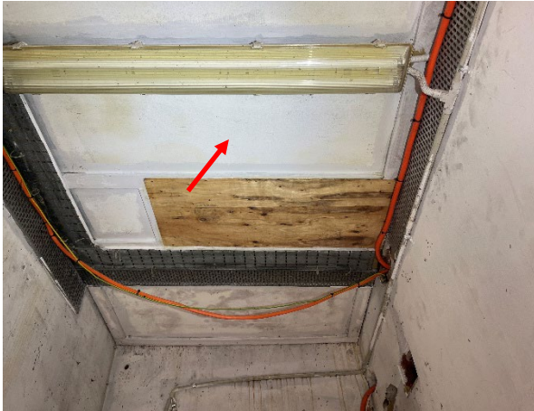
Photo 121: Substation, switchroom, internal, ceiling lining – asbestos containing fibre cement sheeting
