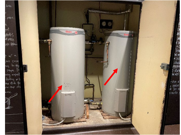
Photo 81: Internal, throughout plant room and tenancies, tanked hot water heater – assumed SMF insulation core
