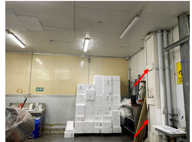
Photo 78: Internal ground floor, Claudio's and Musumeci cool room, structural columns – lead based cream paint
