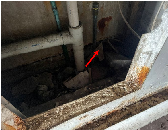
Photo 106: Doyles Warehouse, internal, ground level, central south cool room, wall cavity – asbestos containing fibre cement debris
