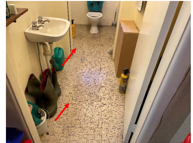
Photo 30: Internal, Net & Tackle, level 1 bathroom floor – asbestos-containing grey vinyl tiles
