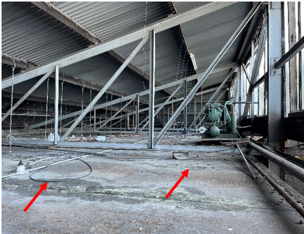
Photo 52: Internal, Poulos Bros above cool room, ceiling cavity – elevated lead concentrations within settled dust
