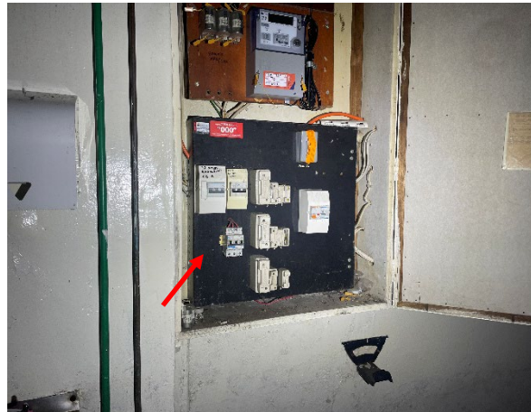
Photo 119: Poulos Bros, internal, ground level, west main room – asbestos containing electrical backing board
