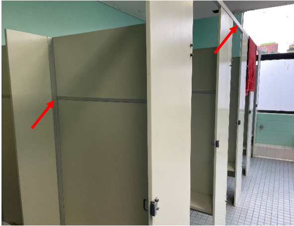
Photo 73: Internal, level 1 northeast staff bathroom, frame to cubical dividers – lead based grey paint
