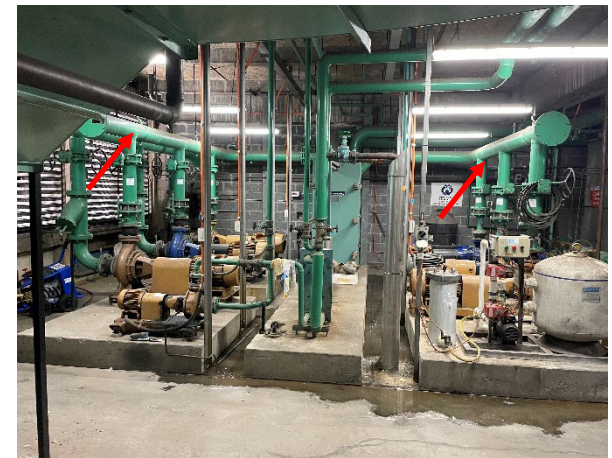
Photo 72: Internal, level 1 plantroom 1, water service lines to water filtration system – lead based green paint
