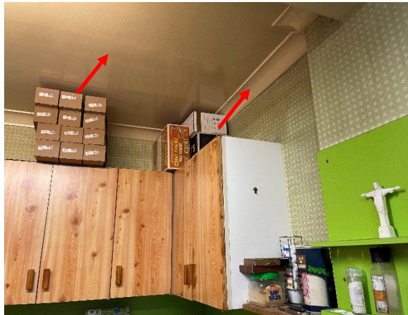
Photo 35: Internal, Net & Tackle, kitchen ceiling – lead based cream paint
