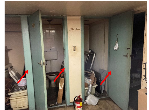
Photo 60: Internal, Salty Squid Level 1, bathroom door and door frame – lead based aqua paint
