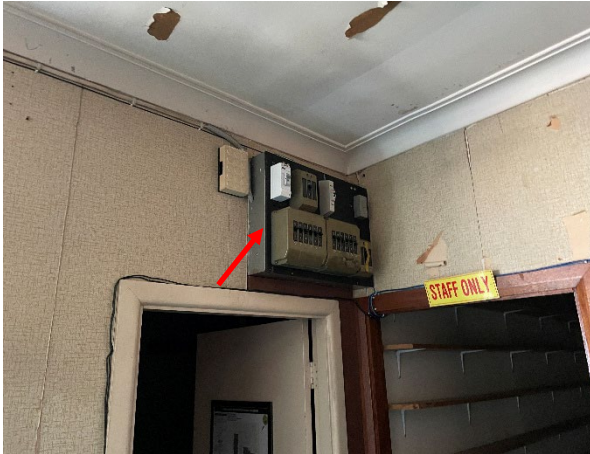
Photo 115: Net and Tackle, internal, level 1, above door to kitchen – asbestos containing electrical backing board
