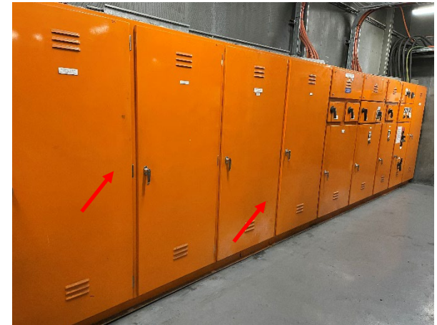
Photo 69: Internal and external, throughout, electrical distribution cupboards and boxes – lead based orange paint
