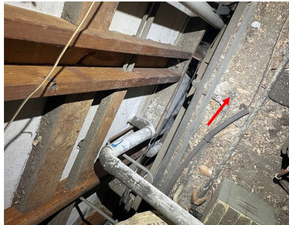
Photo 107: Doyles Warehouse, internal, level 1, wall cavity behind bathroom – asbestos containing fibre cement debris
