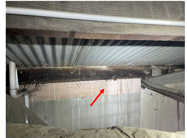
Photo 120: Poulos Bros, internal, cool room, ceiling cavity, infill panel adjacent top of cool room wall – asbestos containing fibre cement sheeting
