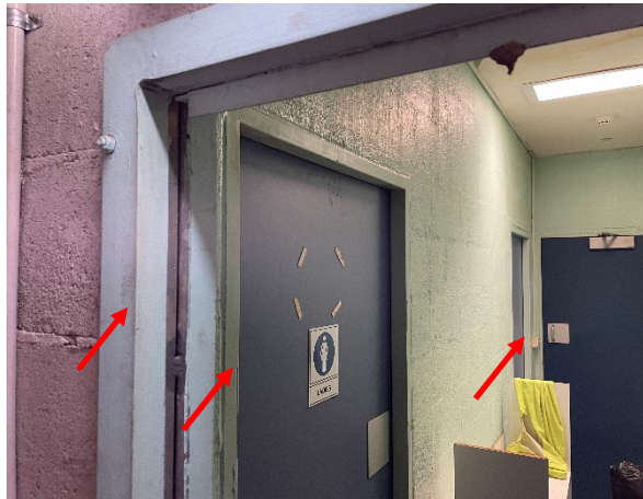
Photo 77: Internal ground level central west, corridor to staff bathrooms and service void for public toilets, door and door frame – lead based blue paint with green overcoat
