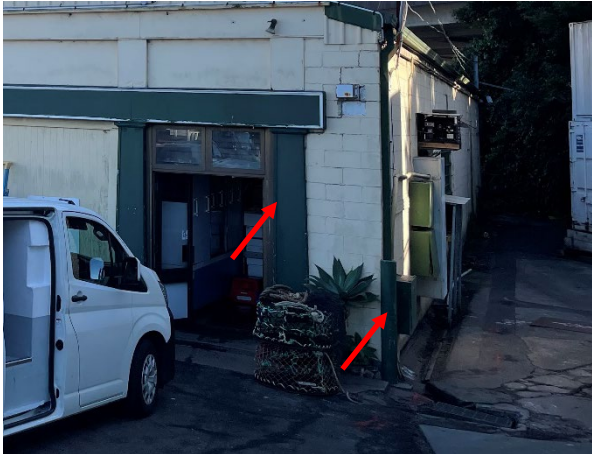
Photo 19: External, Doyle's Warehouse, timber features and traffic bollard – lead based green paint
