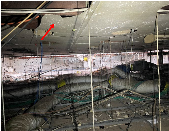
Photo 118: Get Fish, internal, above lining to ground floor, ceiling lining – asbestos containing fibre cement sheeting
