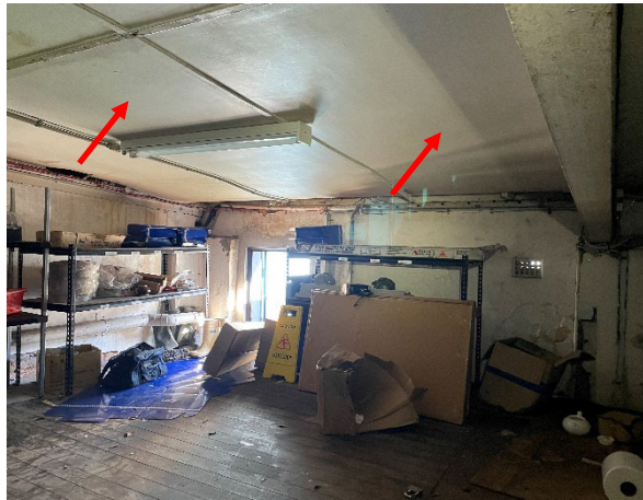
Photo 47: Internal, externally accessed mezzanine level of Sea Emperor, ceiling liner – asbestos containing fibre cement sheet
