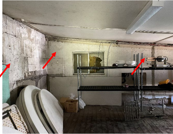
Photo 56: Internal, Sea Emperor mezzanine level, cement rendered brick wall – lead based white paint
