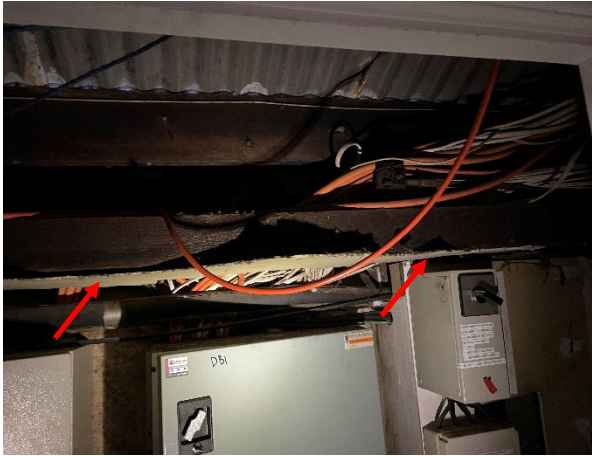
Photo 49: Internal, Get Fish security office electrical cupboard, ceiling liner – asbestos containing fibre cement sheet
