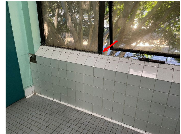
Photo 126: Main Market, external, level 1, north east men's and women's bathroom, windows (assumed to be present to all external windows) – asbestos containing window mastic
