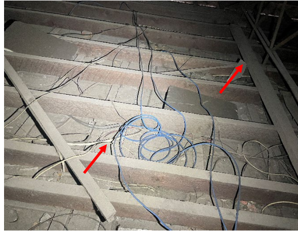
Photo 104: Internal, Doyles Warehouse, ceiling cavity – asbestos containing dust and asbestos containing fibre cement sheeting debris
