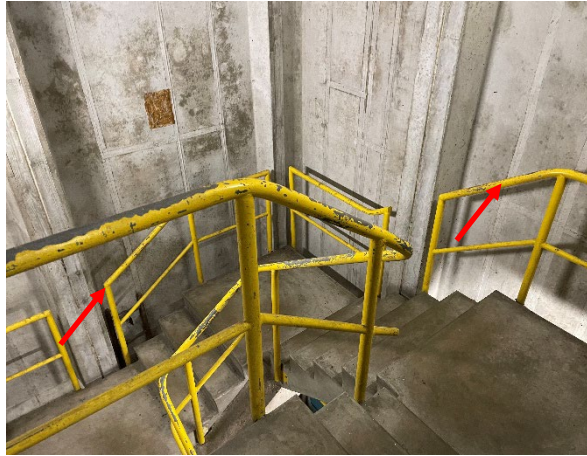
Photo 74: Internal, northeast stairwell, handrail – lead based yellow paint
