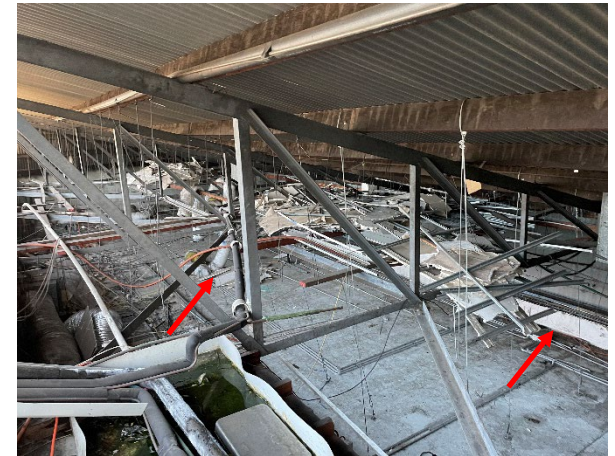
Photo 54: Internal, Get Fish, ceiling cavity accessed via storeroom – elevated lead concentrations within settled dust
