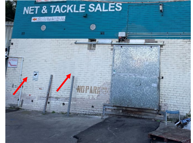
Photo 33: External, Net & Tackle, brick walls – lead based cream paint
