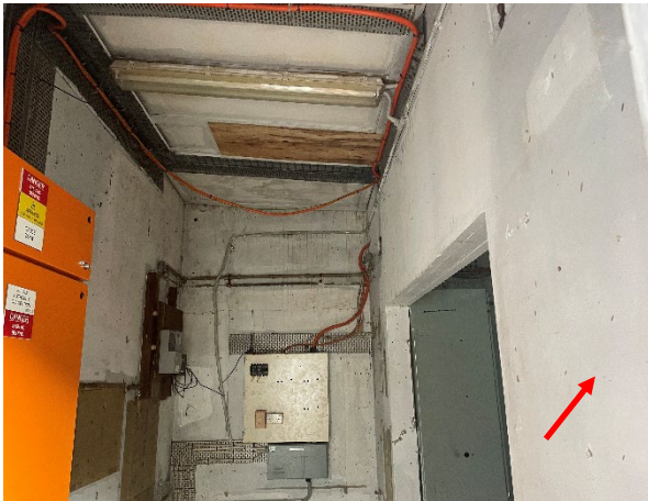
Photo 124: Substation, switchroom, walls throughout – lead based white paint
