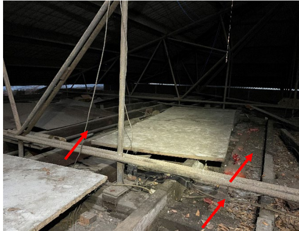
Photo 32: Internal All Seas, ceiling cavity – Friable asbestos and elevated lead concentrations within settled dust
