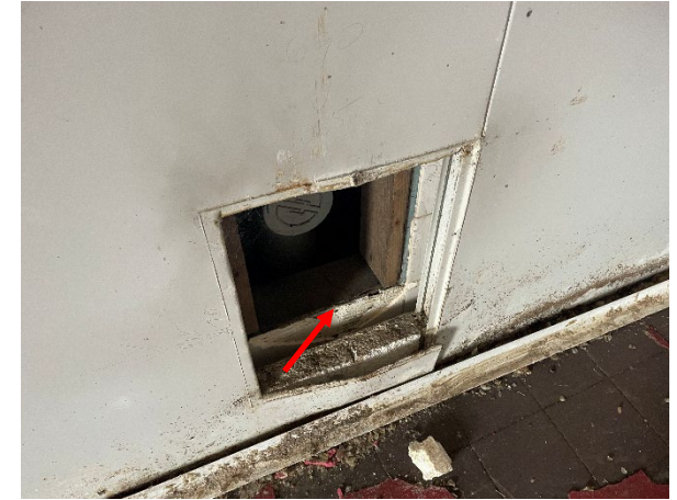
Photo 105: Internal, Doyles Warehouse – ground level central south cool room, behind wall tiles – asbestos containing fibre cement sheeting
