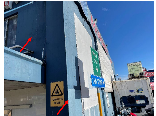
Photo 90: External, wall – lead based blue paint
