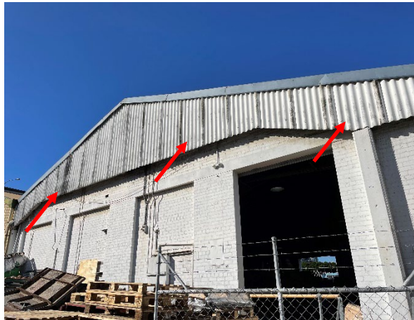
Photo 5: External, Box Recycling Warehouse north gable end – Asbestos containing corrugated fibre cement sheeting
