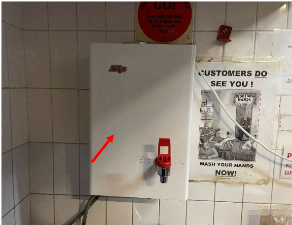
Photo 82: Internal, throughout kitchenettes, Zipp instant boil – assumed SMF insulation core
