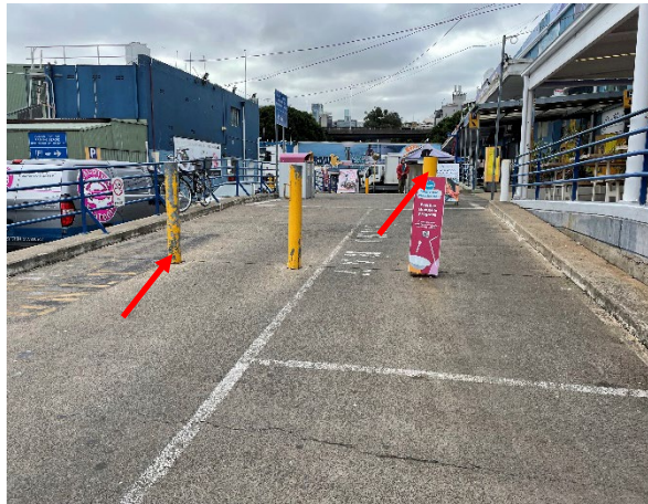
Photo 68: External, traffic bollards – lead based yellow paint
