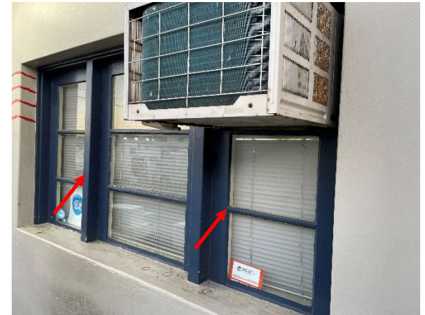
Photo 36: External, All Seas, window frame – lead based blue paint
