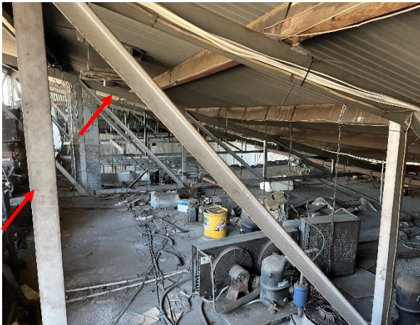
Photo 58: Internal, Get Fish ceiling cavity, meal framework to saw tooth roof – lead based grey paint
