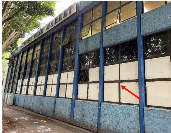
Photo 65: External, east windows, caulking – asbestos containing black mastic
