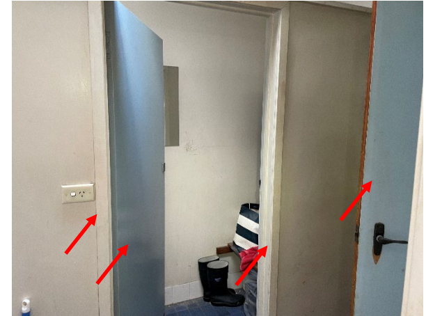
Photo 21: Internal, Doyle's Warehouse, bathroom door and door frame – lead based blue paint with white overcoat
