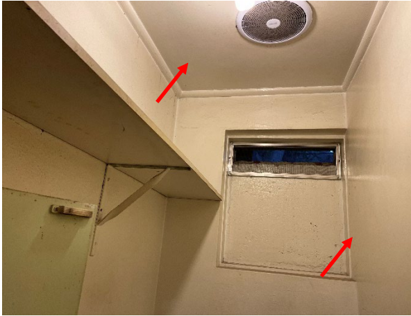
Photo 37: Internal, All Seas, bathroom walls and ceiling – assumed lead containing cream paint
