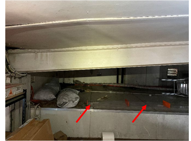
Photo 51: Internal, Sea Emperor above new cool room, ceiling cavity – elevated lead concentrations within settled dust
