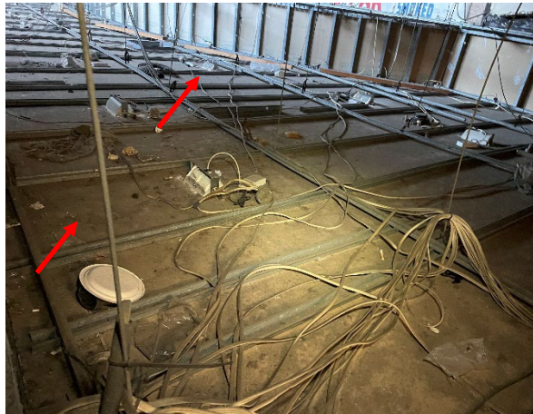
Photo 53: Internal, Salty Squid, ceiling cavity – elevated lead concentrations within settled dust
