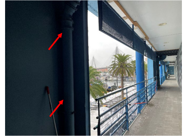
Photo 75: External, level 1 west balcony, cast iron pipework – lead based light blue paint
