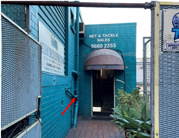
Photo 28: External Net & Tackle, level 1 east entrance, cast iron pipe work – asbestos containing gasket
