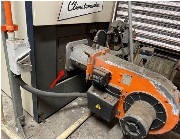
Photo 67: Internal level 1 air conditioning plantroom No. 1, boiler room, Boiler number 2 (north unit) – asbestos containing gasket
