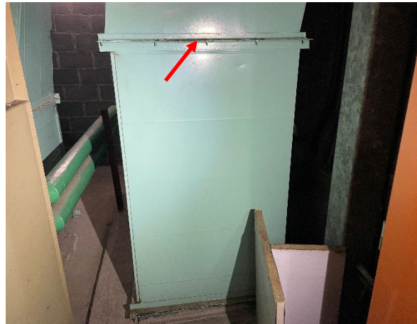
Photo 125: Main Market, internal, level 1, plant room 2, flange joints to air handling unit
